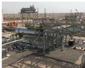
Garraf Gas Treatment Unit Client : PETRONAS Carigali Iraq Holding B.V. Scope : EPC of Gas treatment Unit for Oil-gas Separation Location : Garraf Oil Field, Iraq Execution period : 2013. 11 ~ 2017. 03
